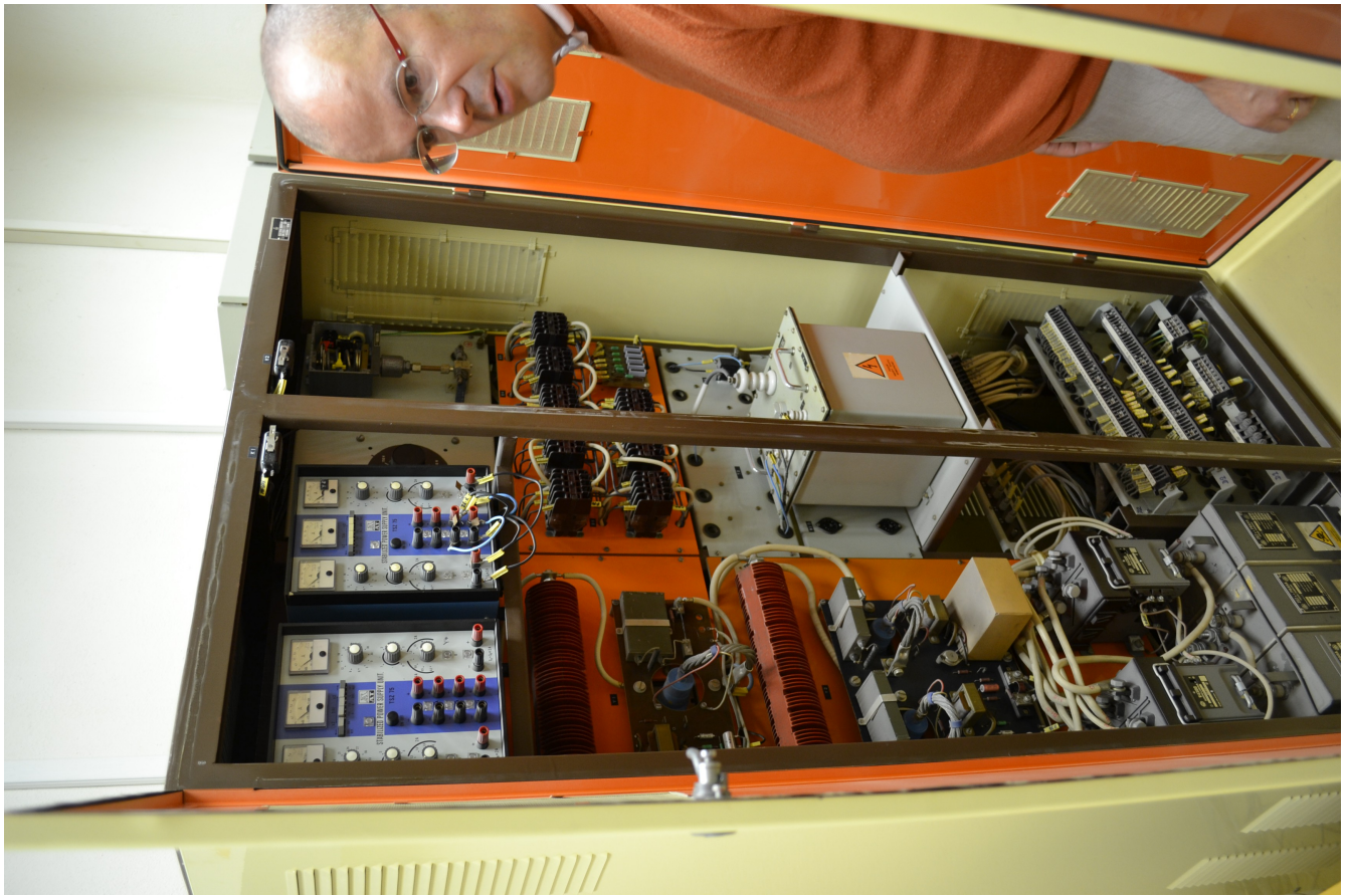
Powersupply and controls for the betatron. Many components are still genuine Czech, manufactured by TESLA.
